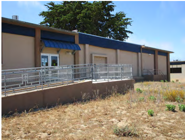
Figure 2. East elevation, rear entrance, awning, and filled in area that originally connected to the multi-story wing, looking northwest. (IMG_0639)
